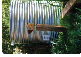
Extensive use of recycled rain water
